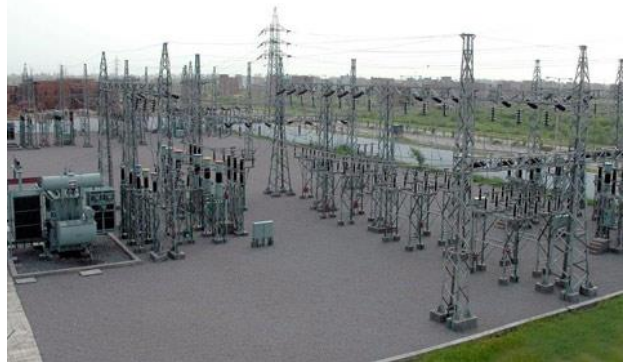
Figure1. Showing 66kV remote controlled Tata Power-DDL Bawana 6 Grid Station
