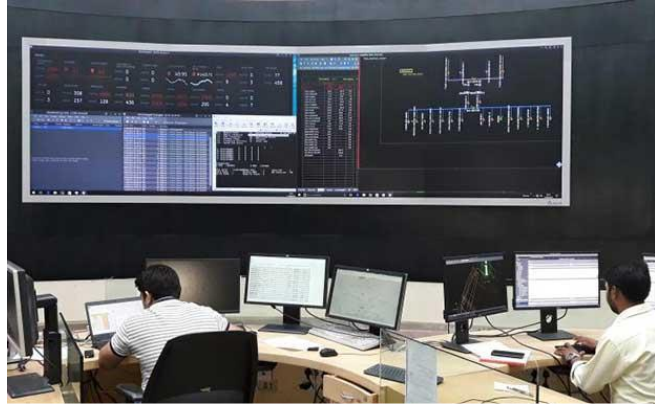
Figure 2. ADMS at Tata Power-DDL
