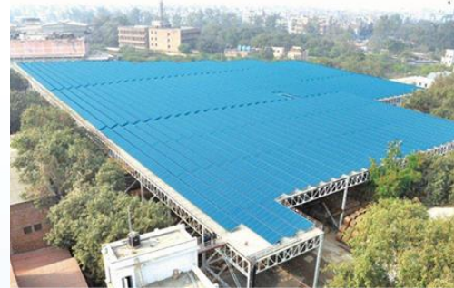
Figure 4. 1 MW rooftop solar PV system at Keshavpuram, New Delhi
