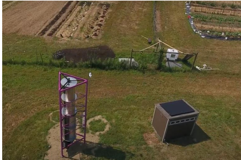
Figure 2: Microgrid with Windstax Vertical Axis Wind Turbine, Solar PV, and Battery Storage.
