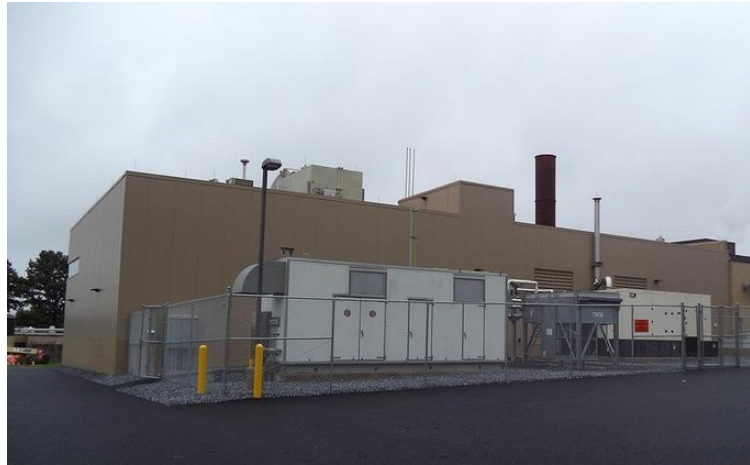
Figure 2: CHP Plant of Milton S Hershey Medical Center
