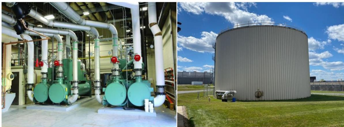
Figure 3: Central Chiller Plant and Chilled Water Thermal Storage Tank at Milton S Hershey Medical Center
