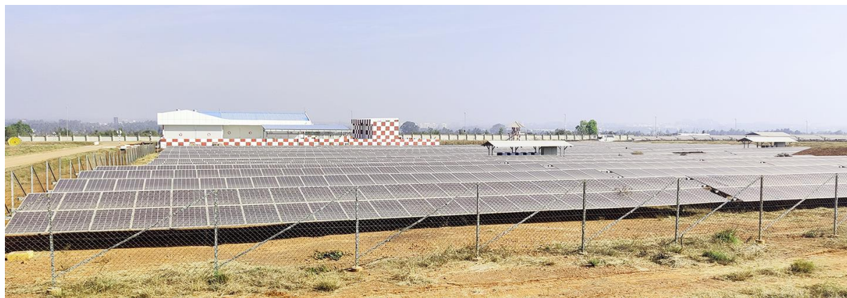
Figure 3: BIAL - Onsite ground-mounted solar PV system
